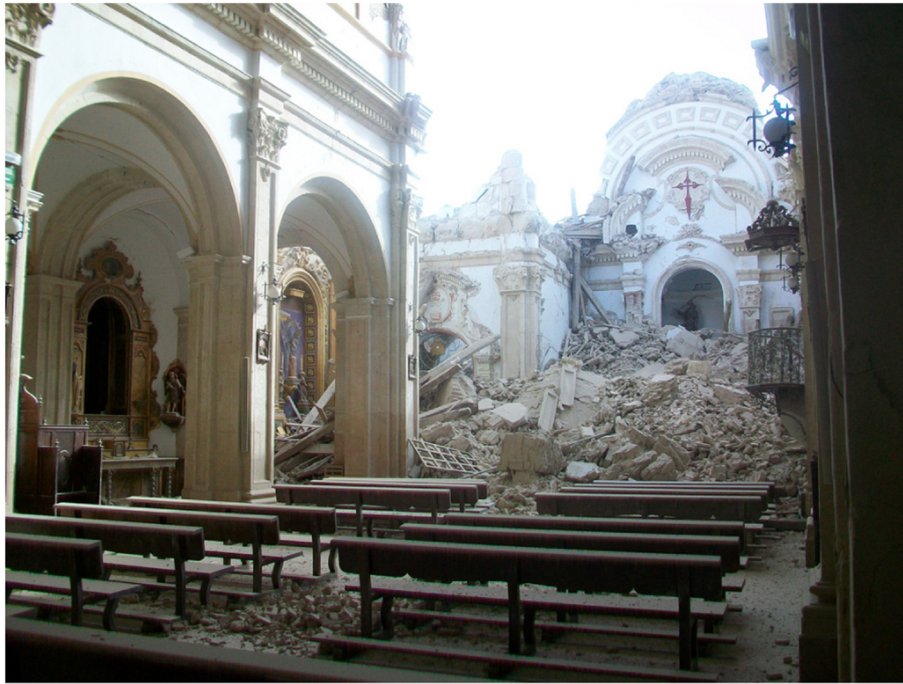
Fig. 14. Destruction in the church of Santiago resulting from the 2011 M_w 5.1 Lorca, Spain, earthquake ( https://en.wikipedia.org/wiki/2011_Lorca_earthquake ).
